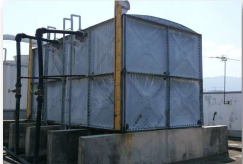
COOLING TOWER MAKE UP TANK
