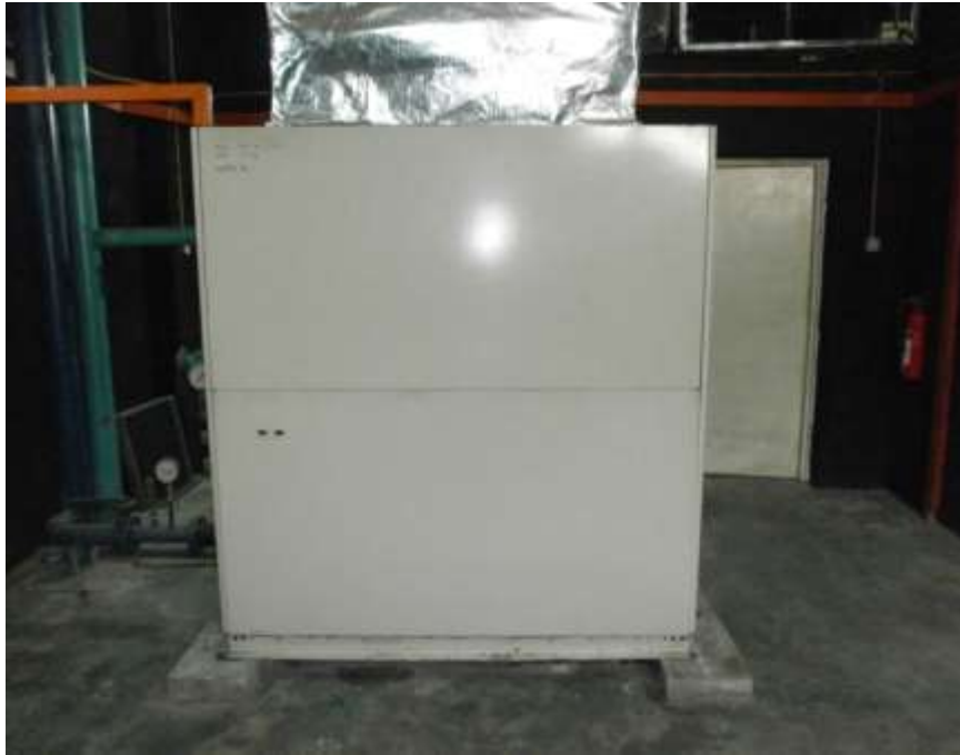
LEVEL 1, 2, 3 & 4 WCPU ( WATER COOL PAKAGE UNIT)
