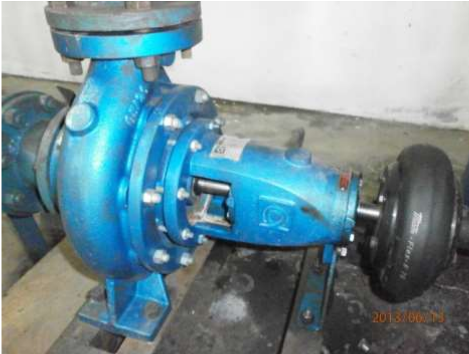
LEVEL 5 CONDENSER WATER PUMP SET (ROOF TOP SIDE A AND SIDE B )
