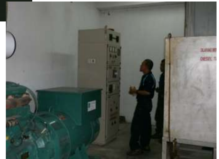
LEVEL 1 GENERATOR SET
