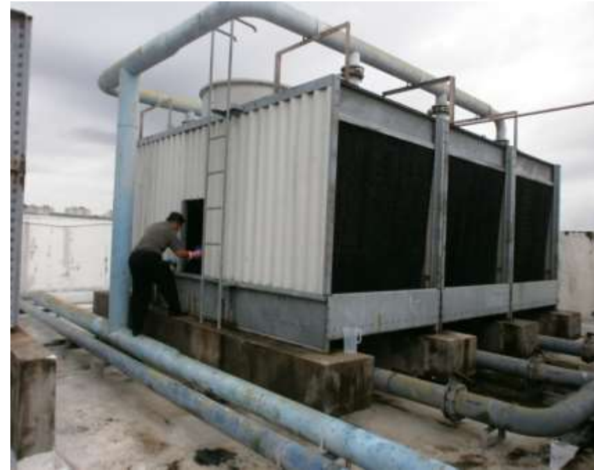
LEVEL 5 COOLING TOWER (ROOF TOP SIDE A AND SIDE B )
