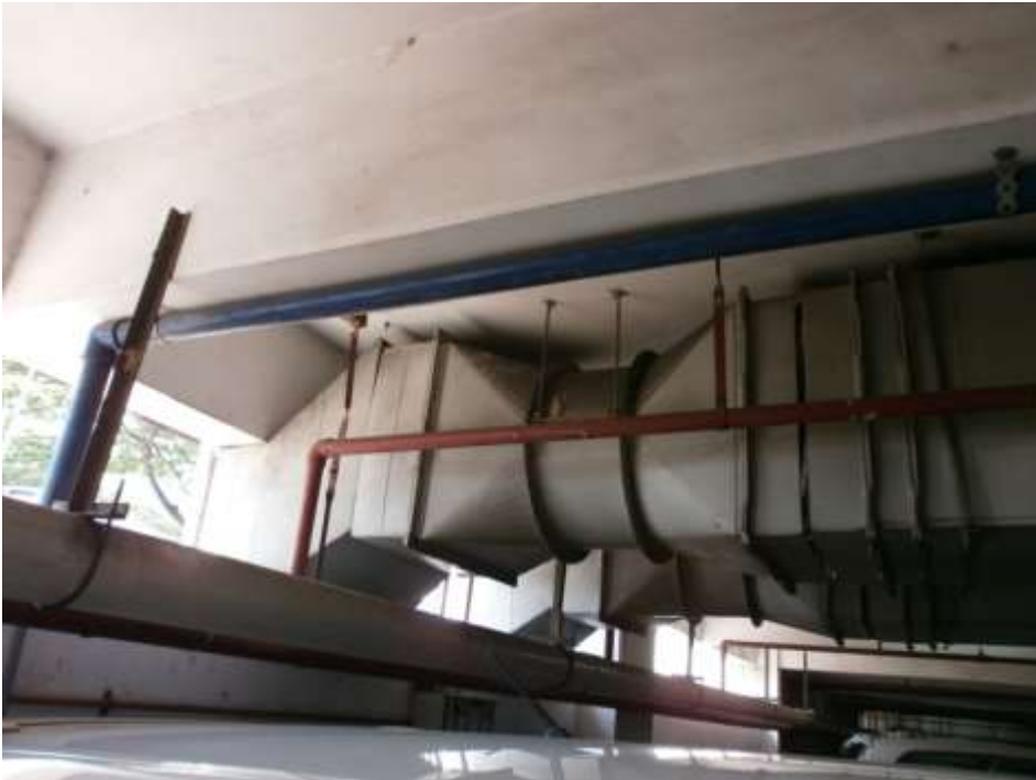
BASEMENT CAR PARK EXHAUST FAN
