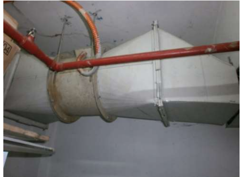
FIRE STAIRCASE FAN – BASEMENT CAR PARK
